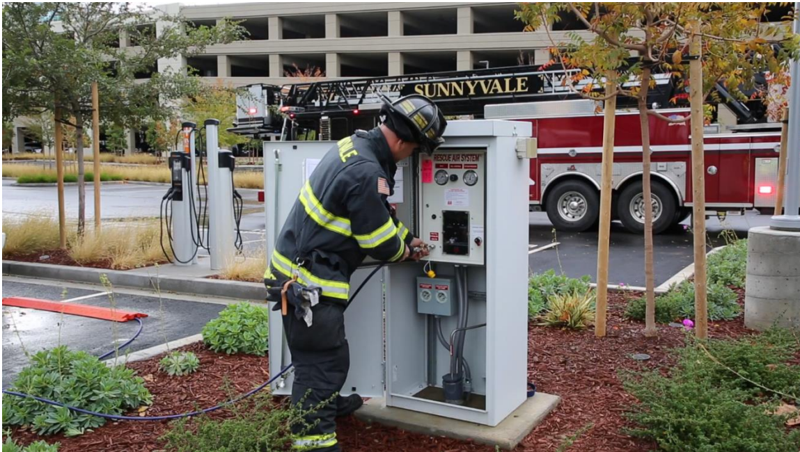
Fig. 2.1: Firefighter connecting MAU to EMAC installed in a remote lockable monument. (Picture: With permission from Sunnyvale Department of Public Safety)
