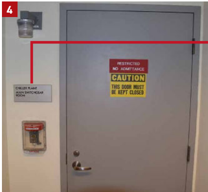
4. A switchgear room label. Note the absence of the term “High Voltage”
